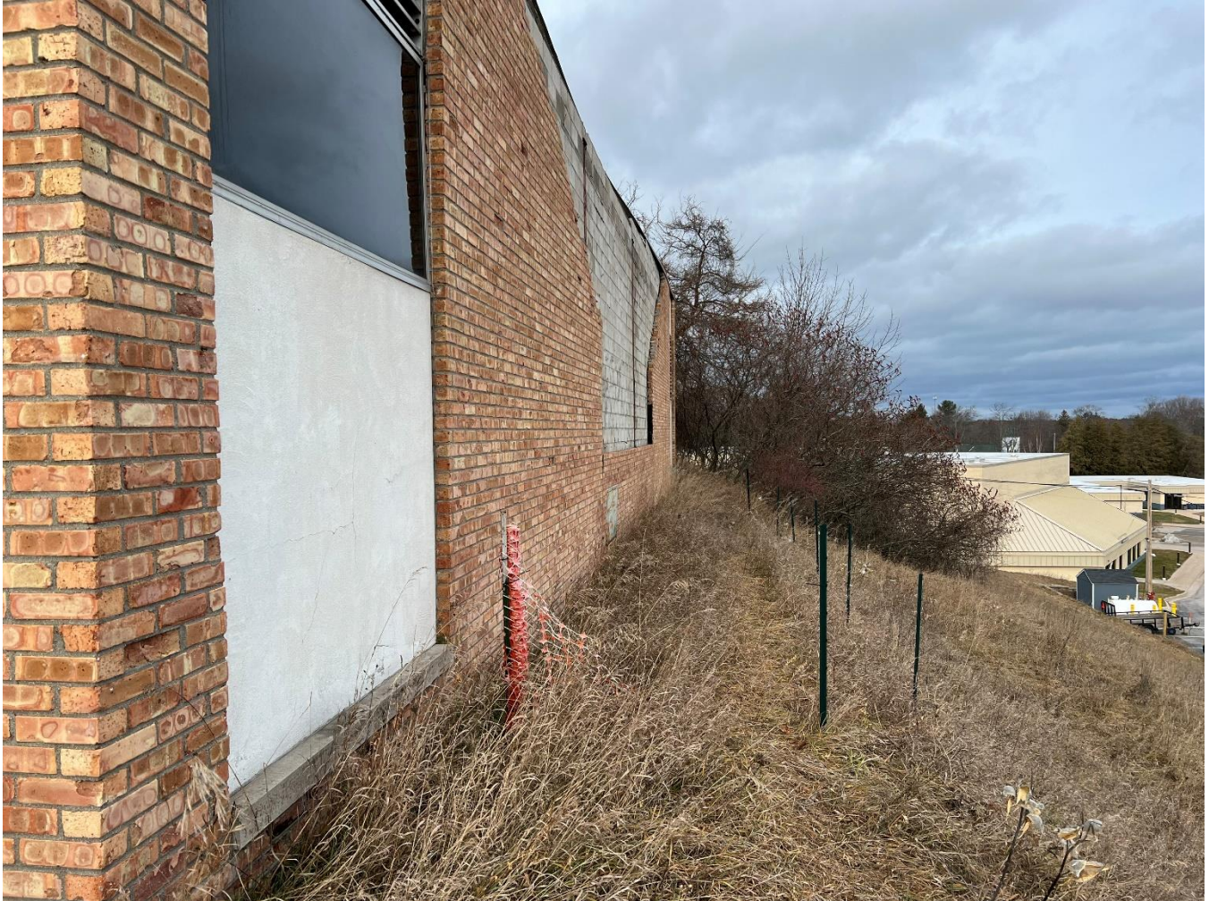
Rear of main building - showing compromised wall and building built into hillside. Northport Public Schools building is background of photo (north of main building).
