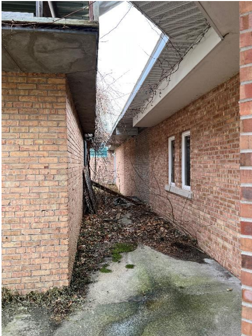
Close Proximity of buildings Left -Main Bldg to demo; Right – Highlands (preserve)
