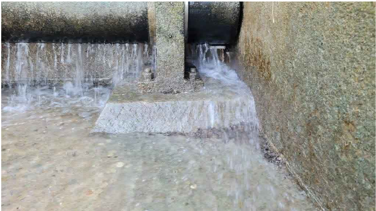
Seepage through Gate While in the Closed Position on the Left Side
