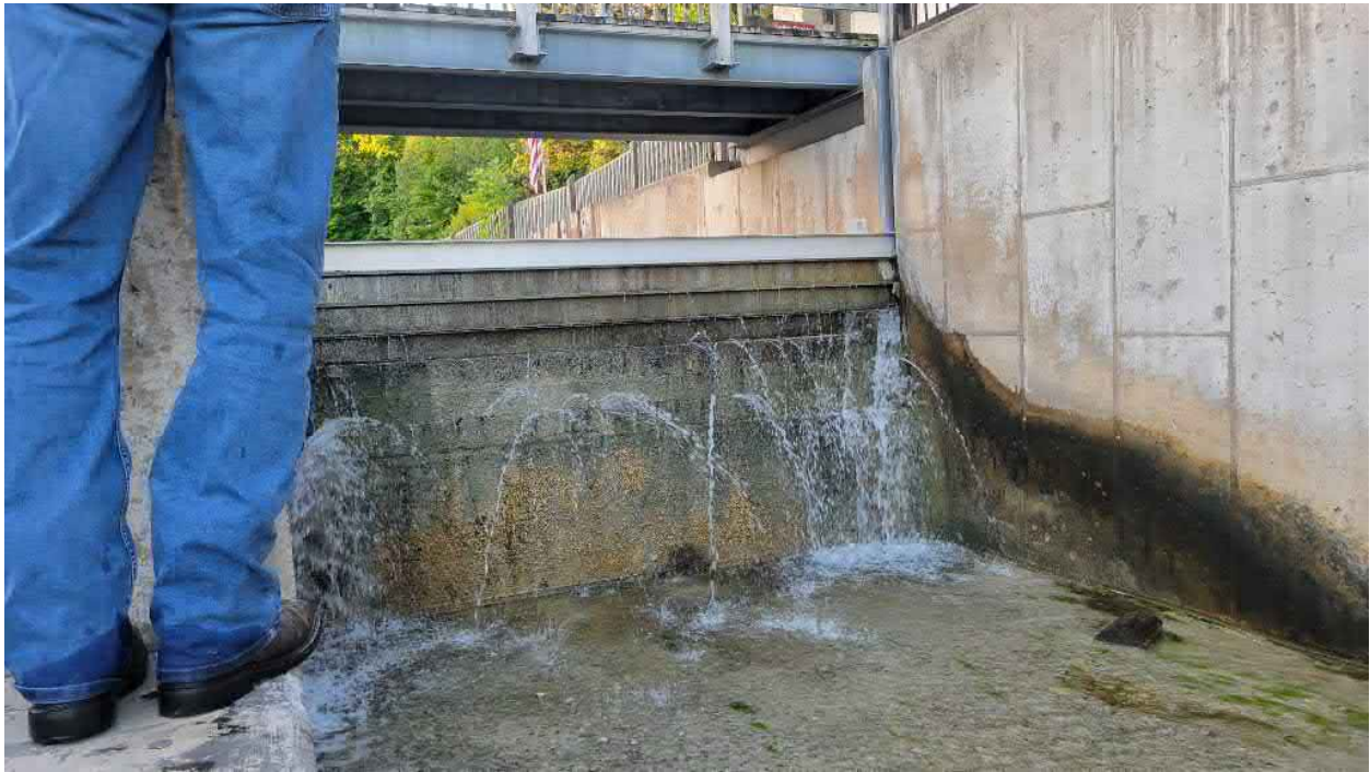
Seepage between Boards of Auxiliary Spillway
