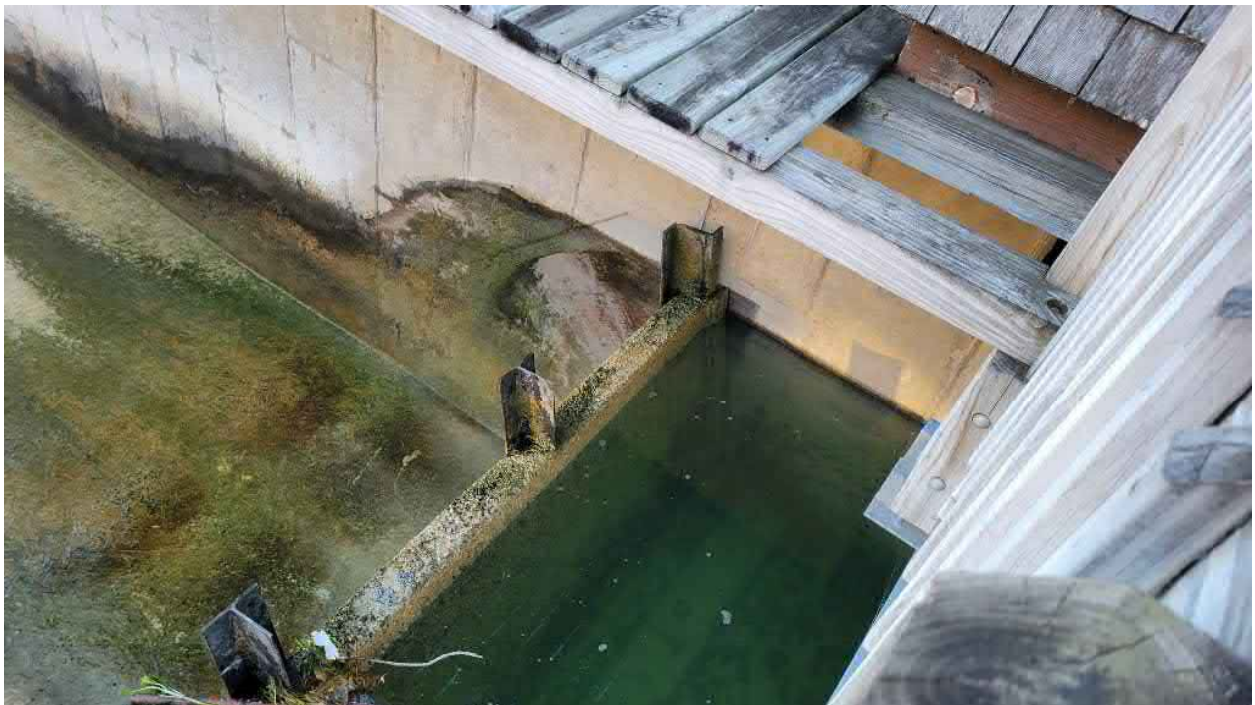
Closed Hydraulic Gate (Right Side)
