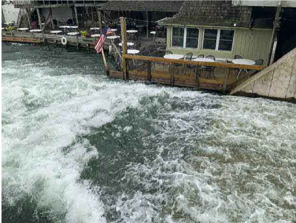
Looking north at downstream end of principal spillway and downstream end of right principal spillway abutment wall.
