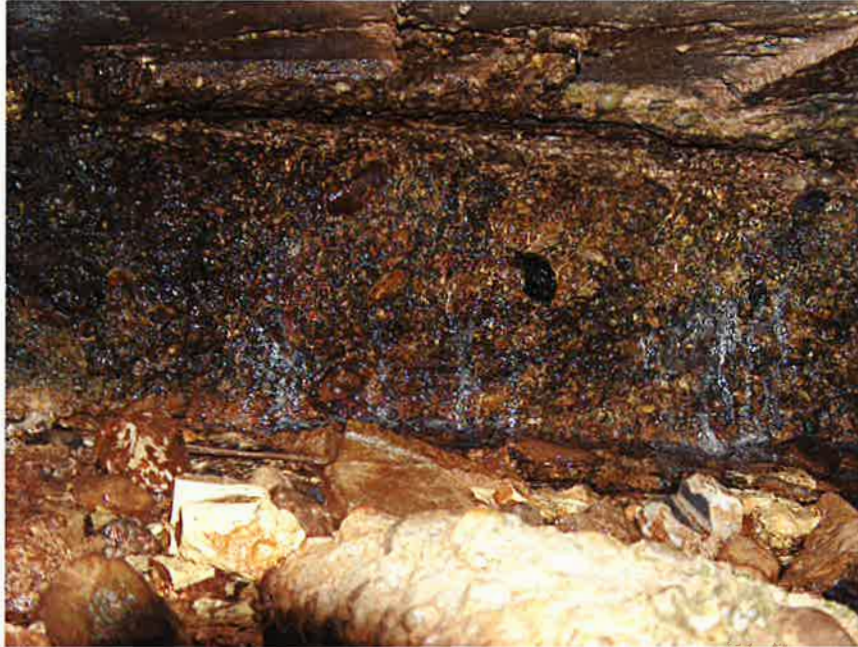
Photo 7. View of seepage flow from under DS right (south) side of spillway slab, 2003 photo.
