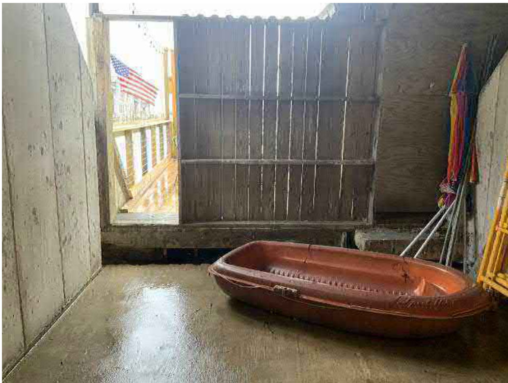
Looking downstream from just downstream of main door into hydraulics / control room.
