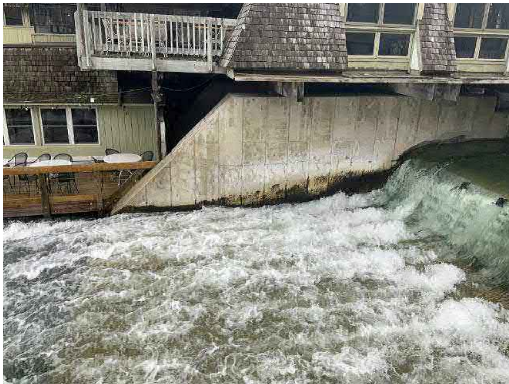
Looking northeast at downstream end of principal spillway and downstream end of right principal spillway abutment wall.
