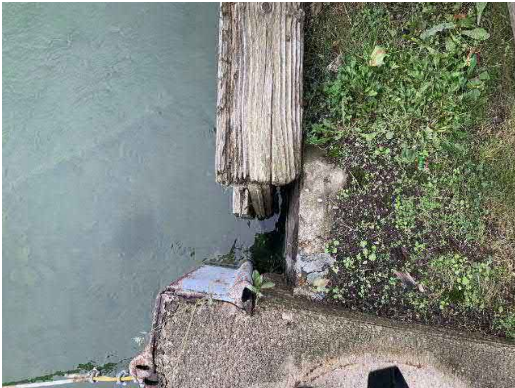
Left approach abutment wall upper end at northwest end of wood seawall.
