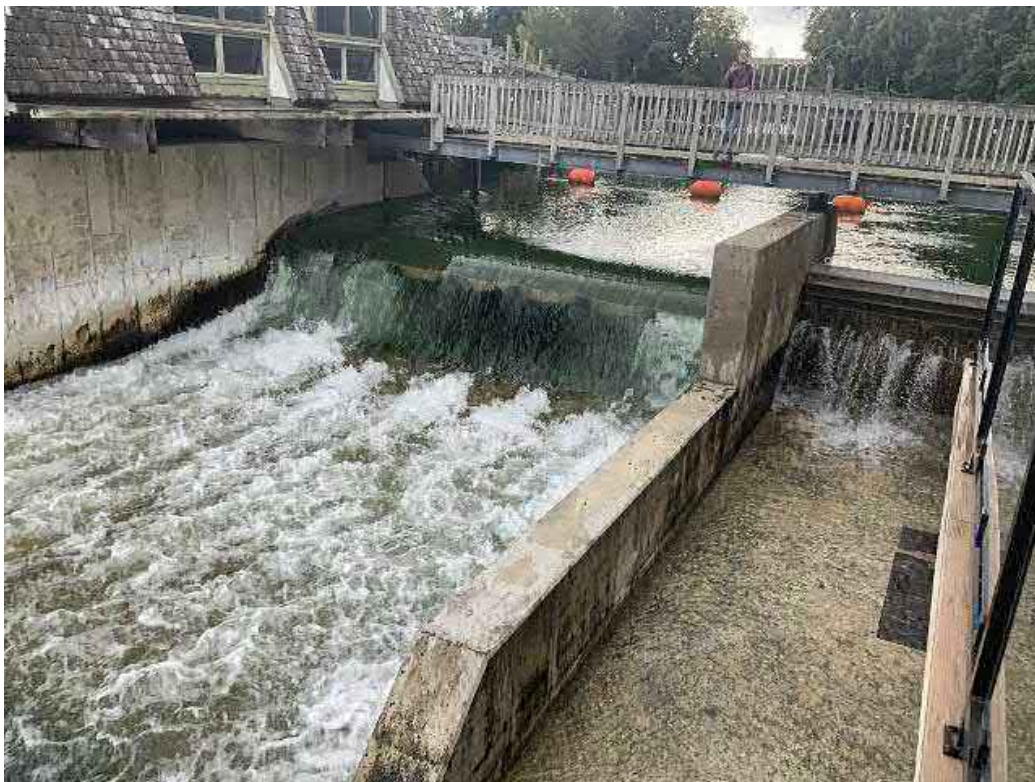
Looking southeast at Principal (former Bay #2 and #3) and fixed crest / stoplog (Bay #1) spillway.
