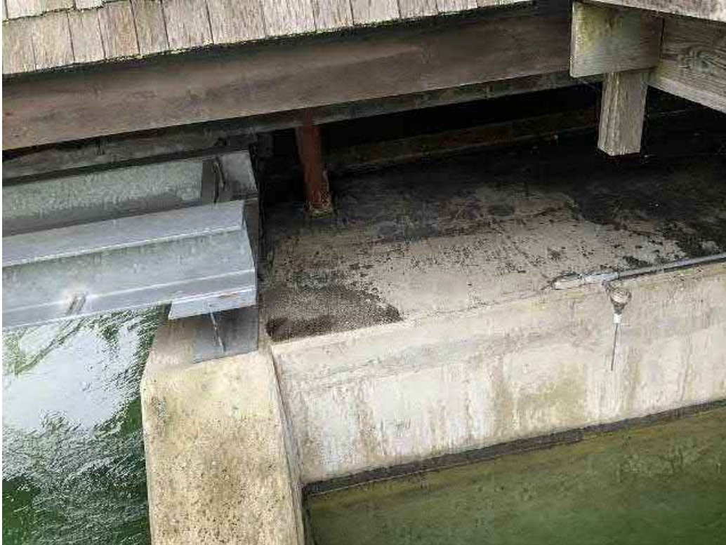
Upstream face of concrete wall and roof at hydraulic / control room (former Bay #4) Walkway steel I-beam supports.
