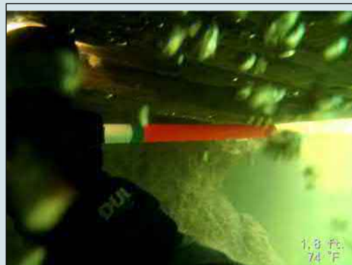
Downstream spillway overhang
