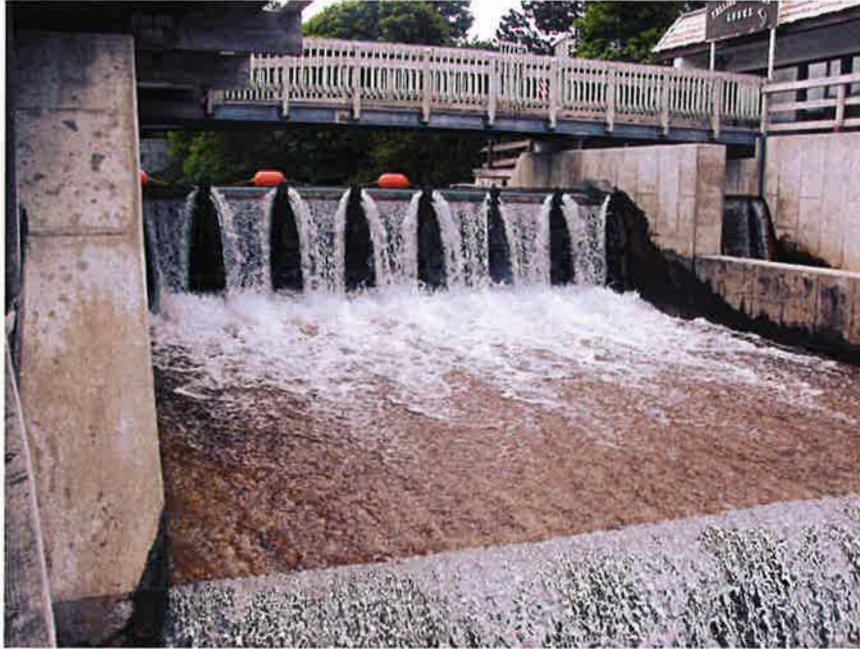
Photo 3. DS view of primary crest gate spillway and operators/access bridge. Gate at legal summer level.
