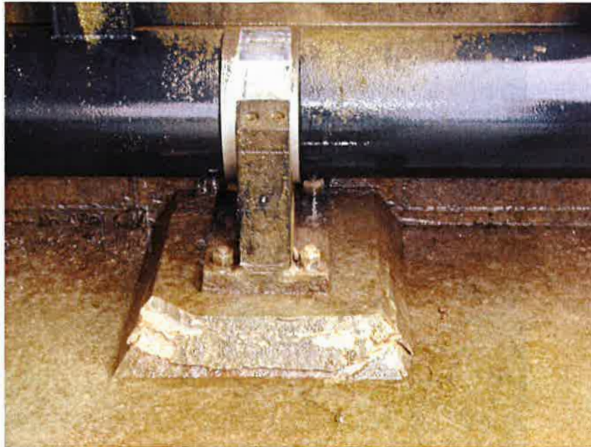
Photo 5. View of spalled grout gate bearing pad.
