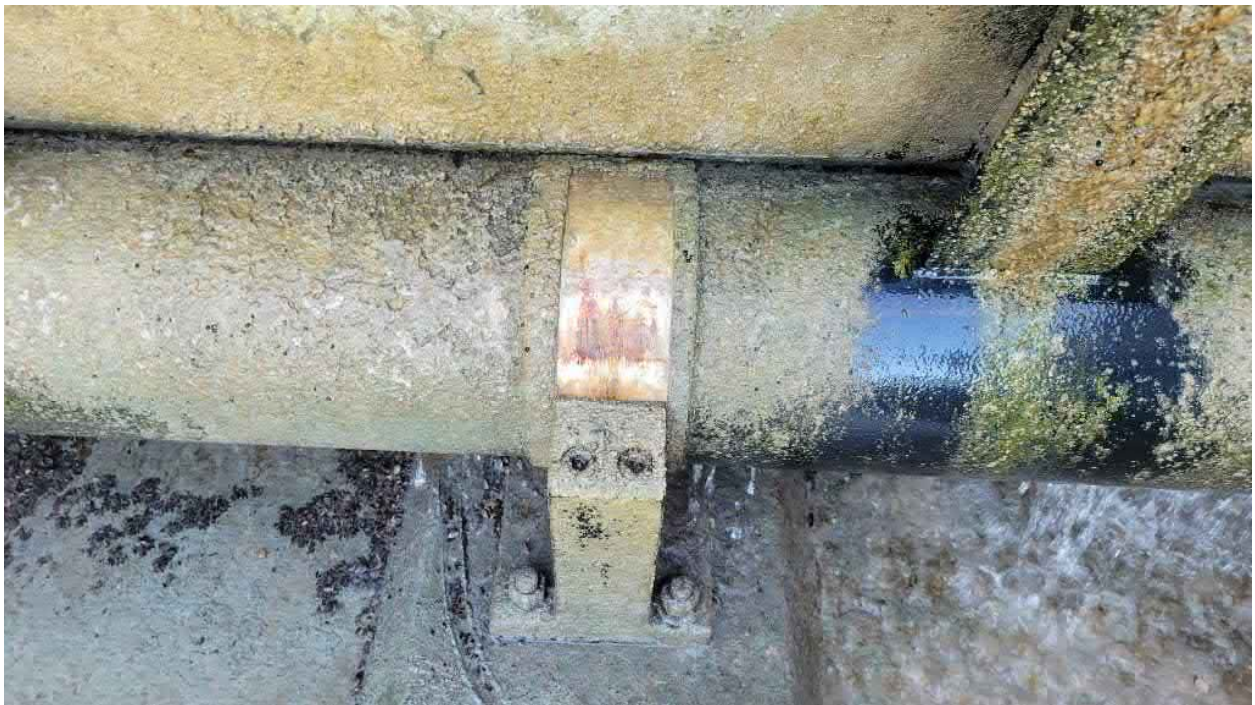
Joint Observation - Corrosion
