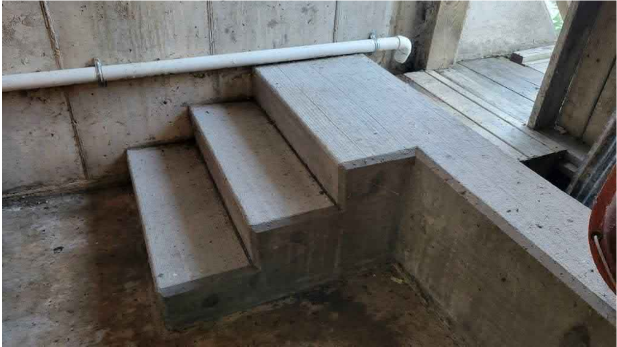
Control Room - Concrete Curb Flood Protection
