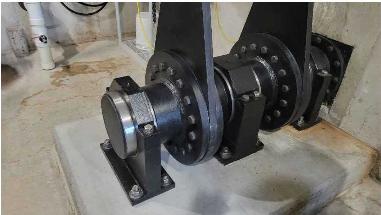
Shaft Connection to Hydraulic Lift
