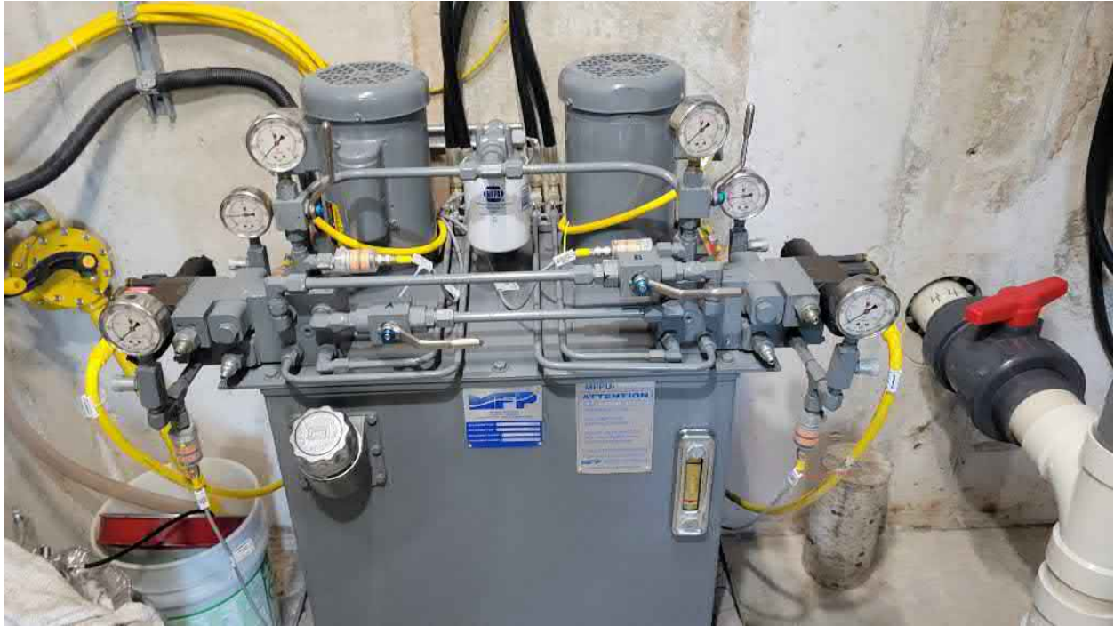
Control Room - Hydraulic Reservoir and Pumps
