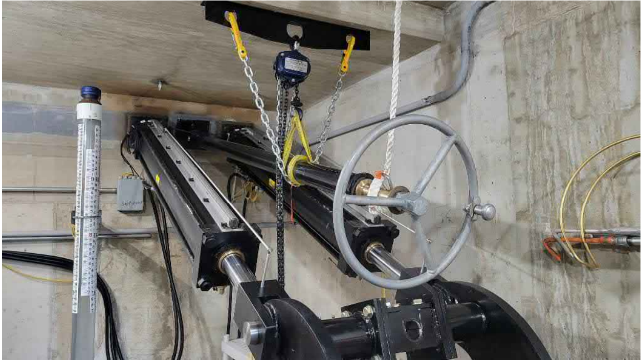
Installed in 2020 - Manual Operator for Hydraulic Lift
