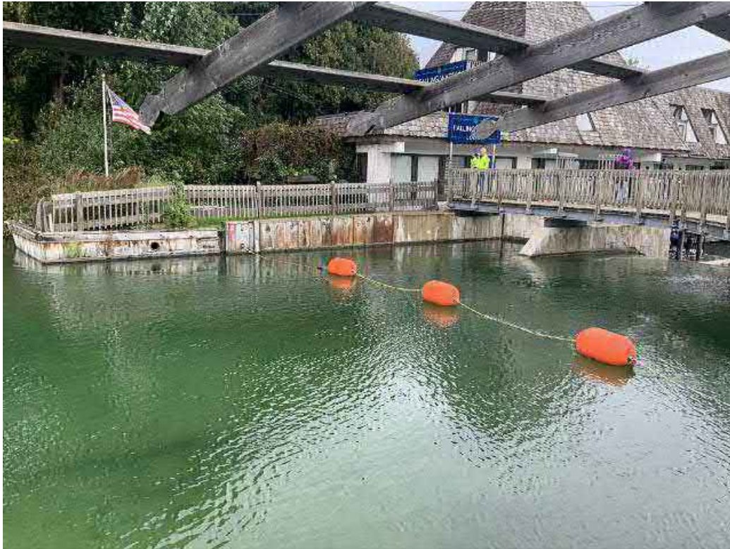
Looking southwest across upstream face of dam at left upstream abutment wall and wooden seawall fence.
