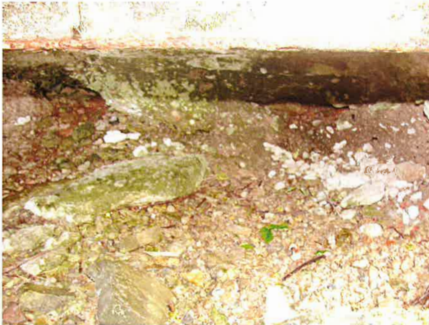
Photo 8. View from under DS right (south) side of spillway slab, 2012 photo. No seepage.
