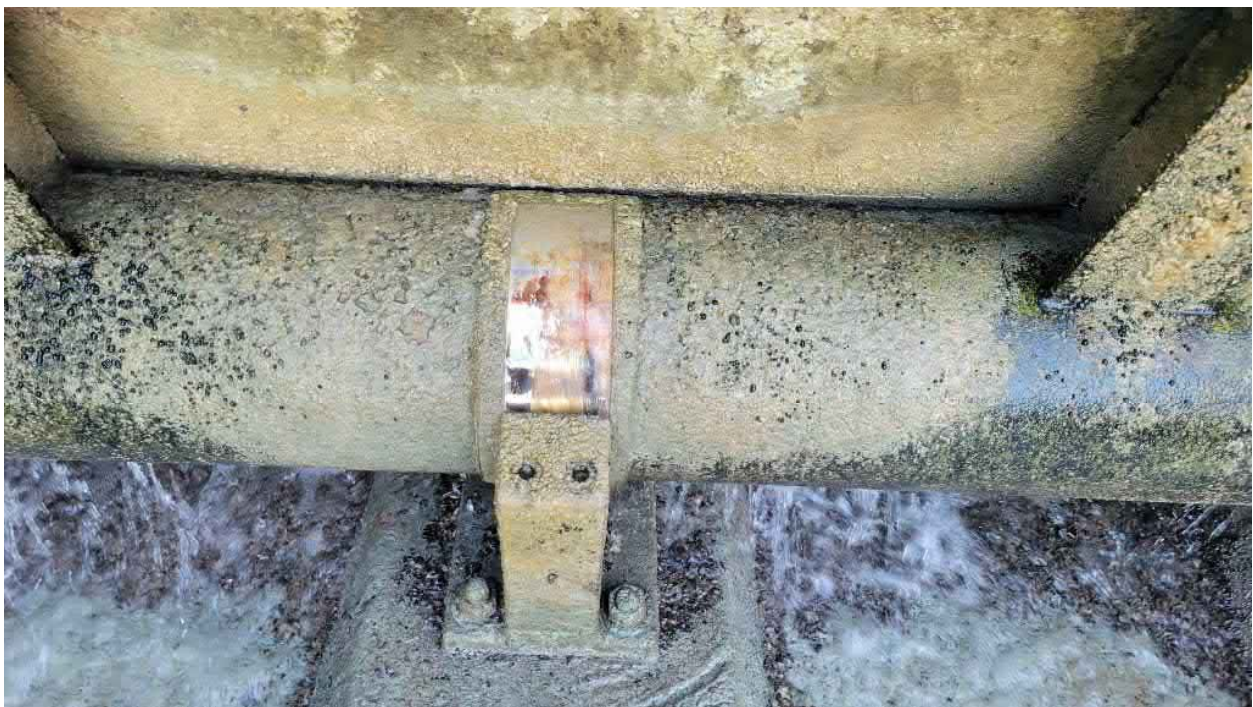
Joint Observation - Corrosion
