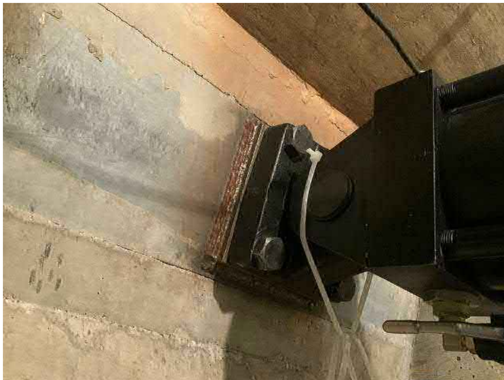
Hydraulic ram mounts to steel I-beam at ceiling / wall corner (typical of 2).
