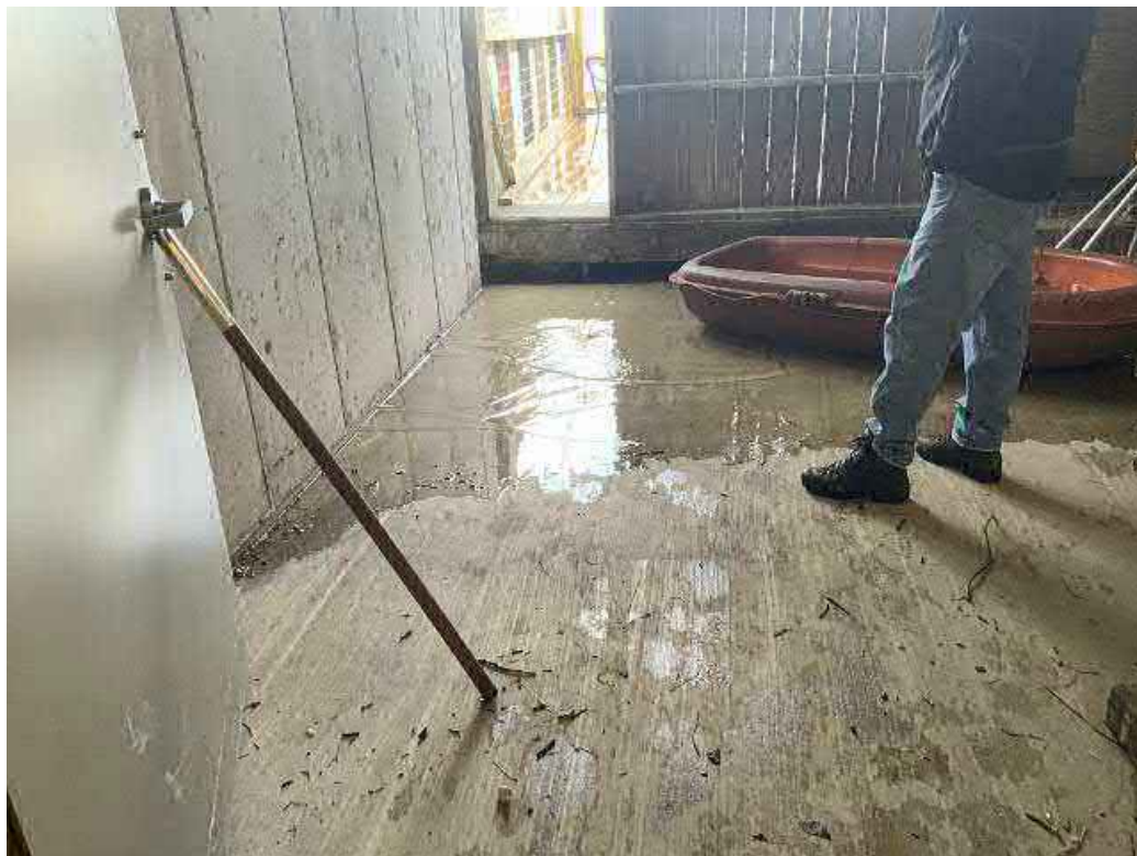
Typical backflooding into Bay #4 downstream of hydraulic / control room due to high Lake Michigan water levels.
