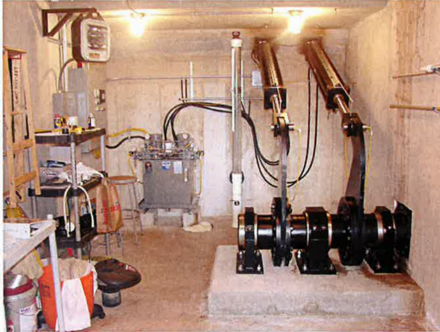
Photo 9. View of automated control panel, hydraulic system, dual rams, gate torque arms and end bearing, and headwater sensor in operations control room.
