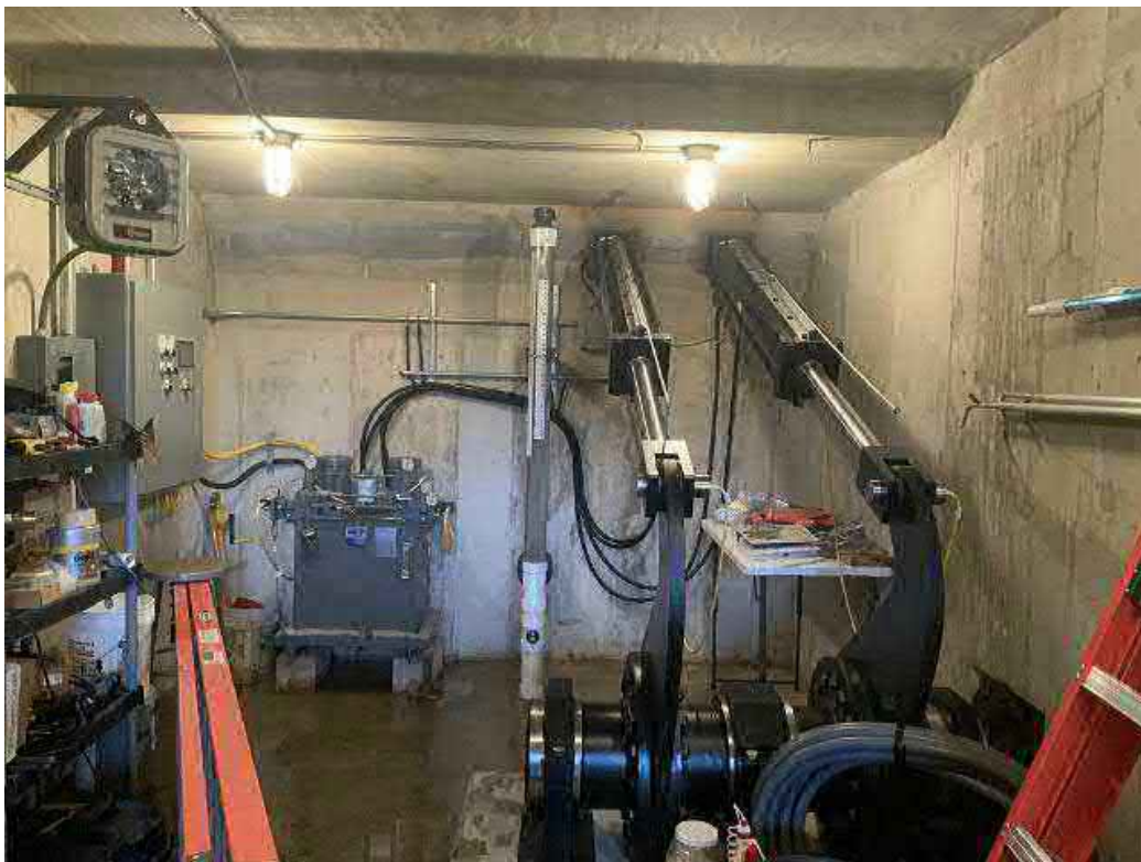
Looking southeast within hydraulics / control room at hydraulic gate actuators.
