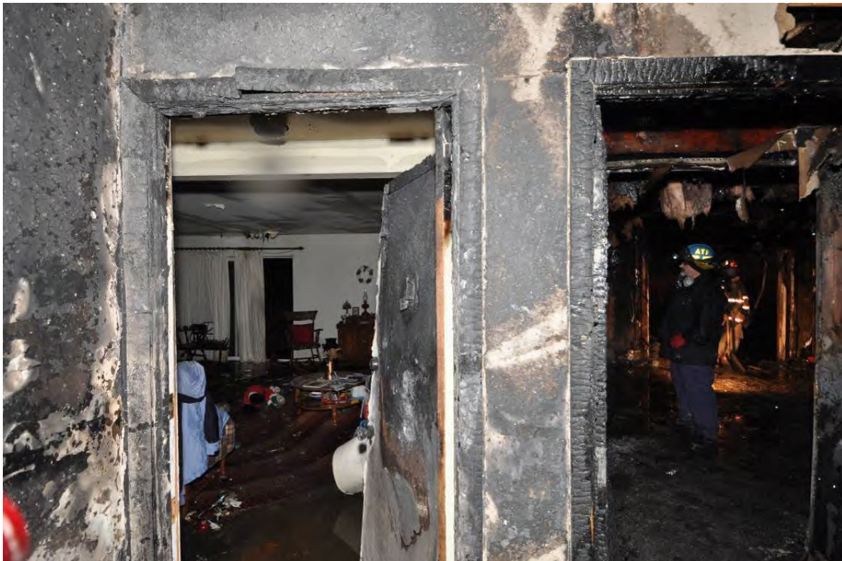
This picture depicts the effects a fire has on rooms with an open door and a closed door.
