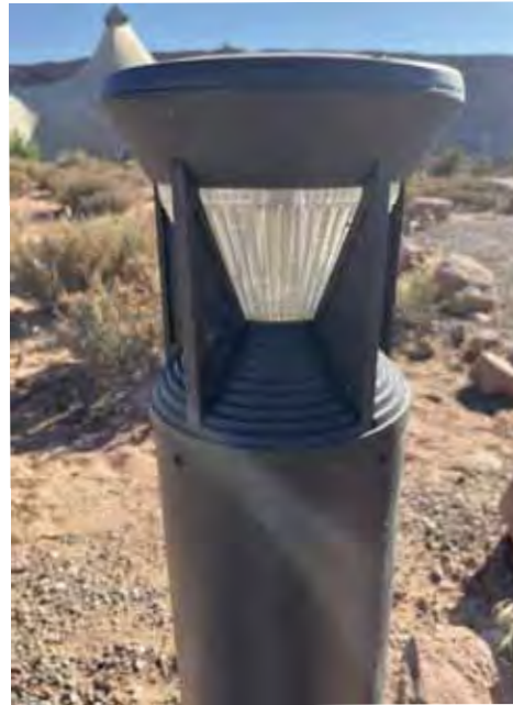
Figure 3 Driveway Bollard Lighting
